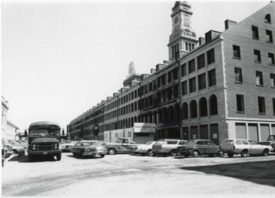
Figure 23. South Market undergoing rehabilitation, 1975. View east. Source: Courtesy of U.S. Department of the Interior, National Park Service.
