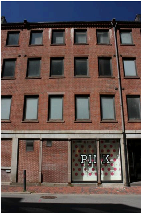
Figure 17. South elevation: Typical building unit with atypical cast iron pilasters at storefront.
